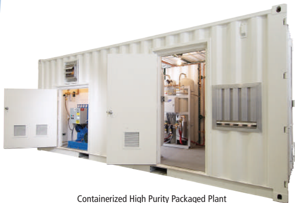
Containerized High Purity Packaged Plant
